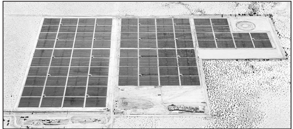
Blythe Solar Power Project, Blythe
